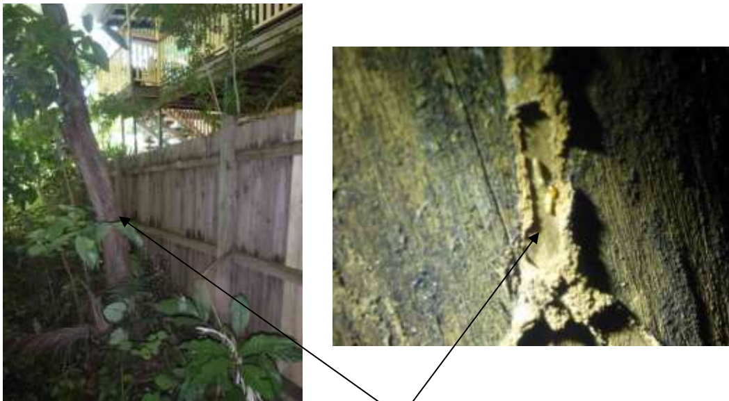
Live termites in workings
